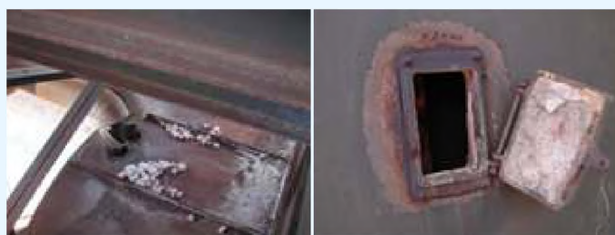
Figure 4: Tramp Air Leakage a) Tube Penetrations b) Open Sight Port
