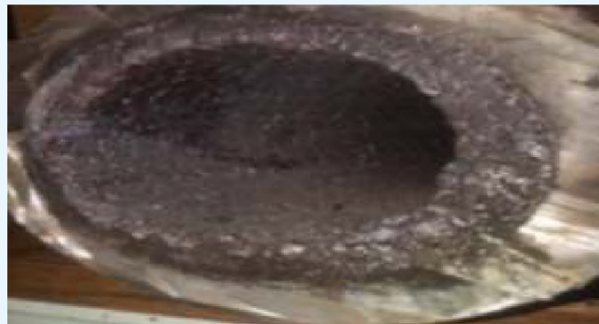
Figure 7: Accelerated fouling at reduced load
