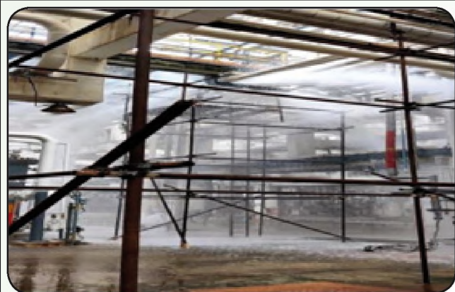
Figure 3: Before Leak Arresting
