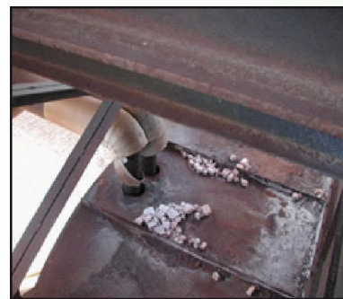
Figure 6.0: Tramp air through tube penetration
